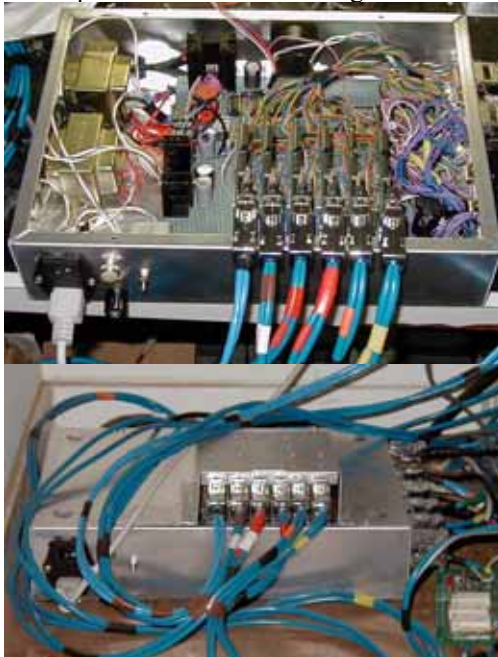
Figure 2. Controller (A) innards. (B) Buttoned up and operating. There are many more wires beneath the board!
