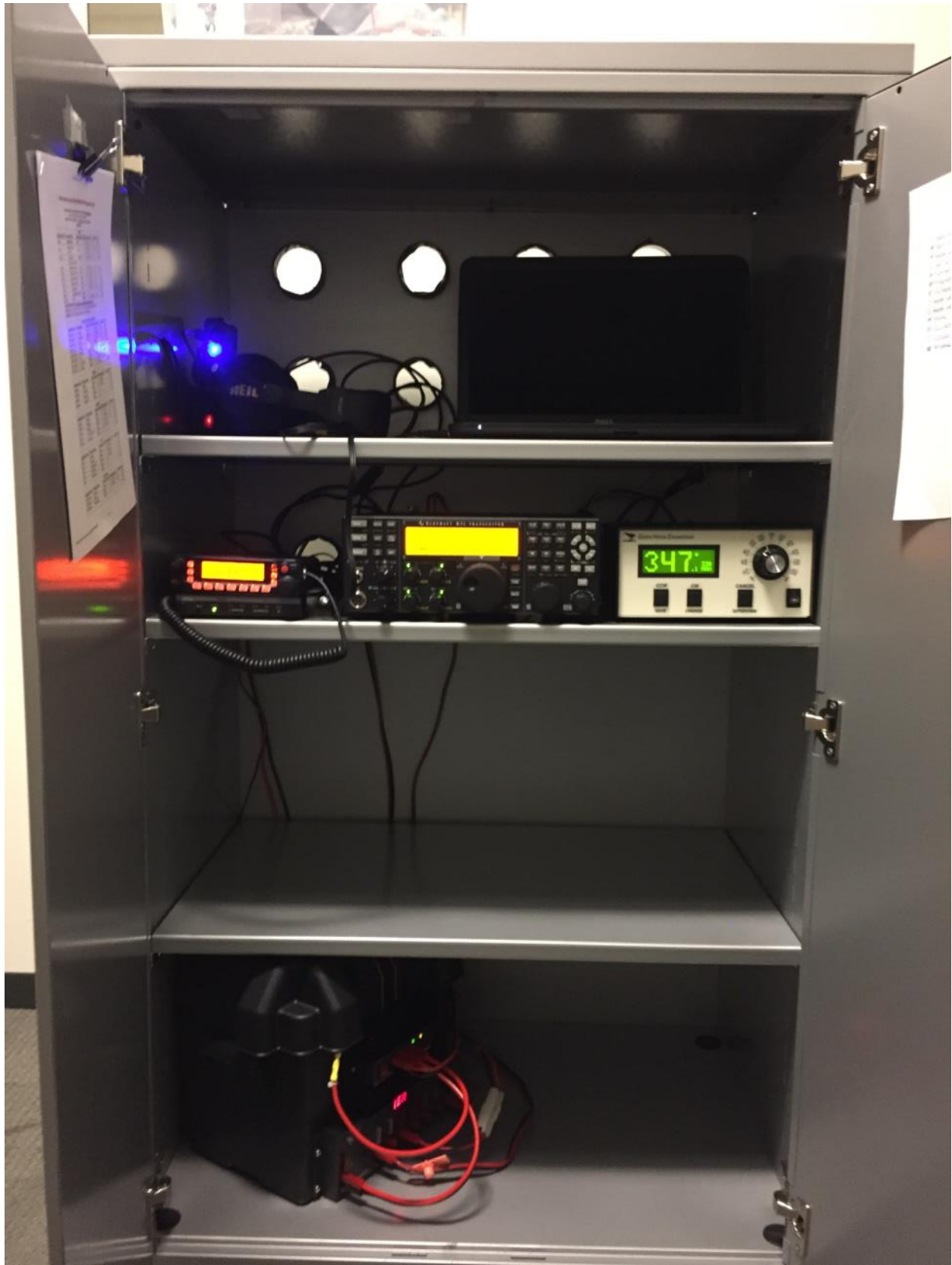
Inside the W6VMW cabinet
