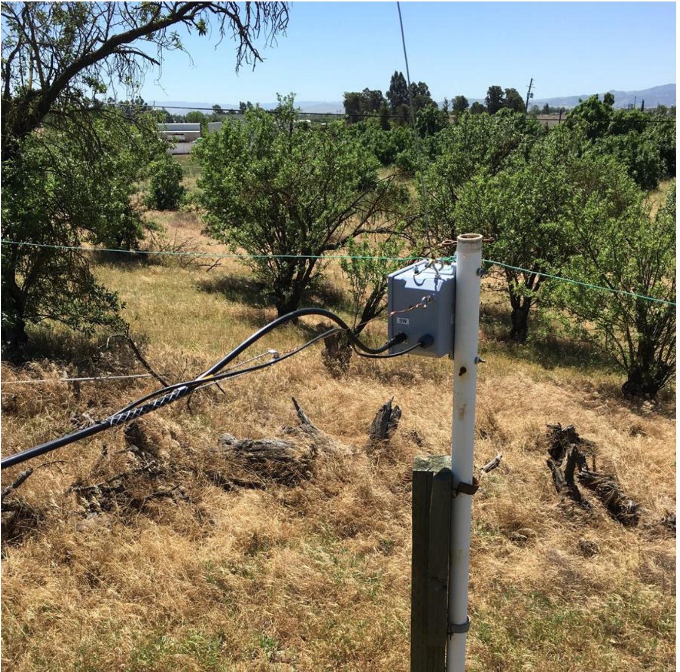
Figure 4. Antenna box installed. Feedlines have nice strain reliefs. This should hold up well. If only the wires would survive all that flexing the wind.
