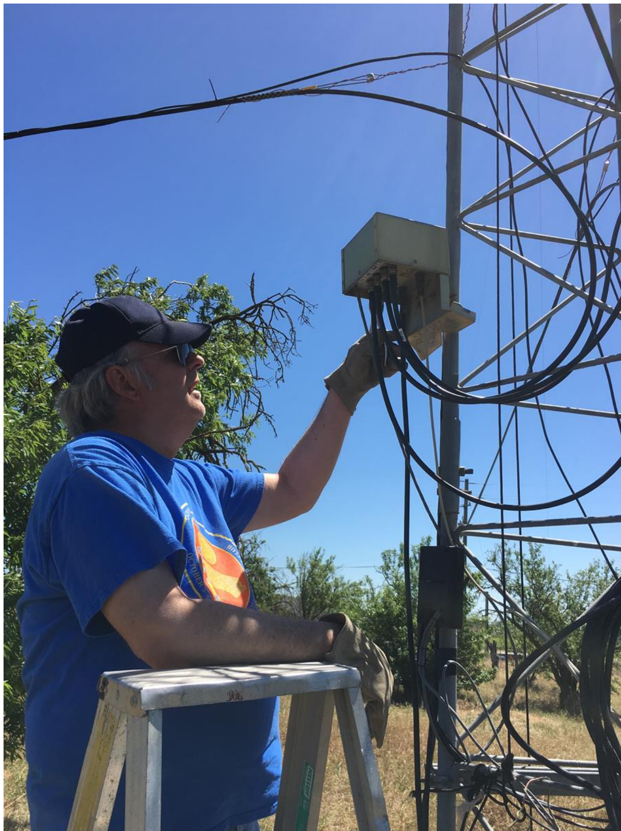
Figure 6. Lee KI6OY attends to the Comtex box. SO-239s get a coat of Dow DC4 dielectric grease, and a good tightening.
