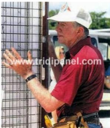
Pres. Jimmy Carter installing TriD panels on a housing project for Habitat for Humanity
