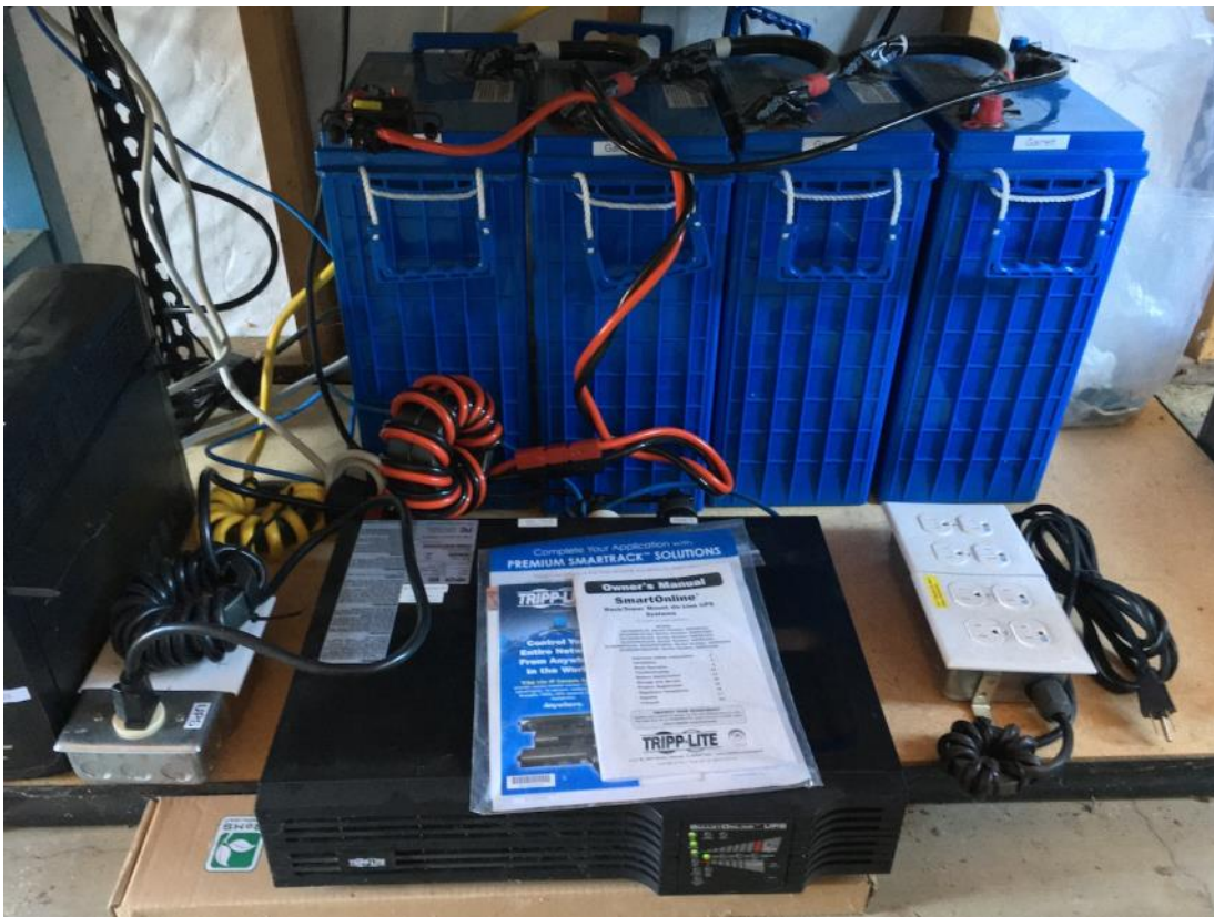
Figure 4. The second UPS installation, with all filtering devices visible.
